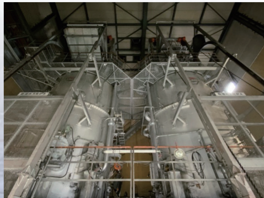
Dry distillation gasification incinerator
