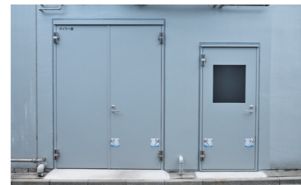
Water stop door
